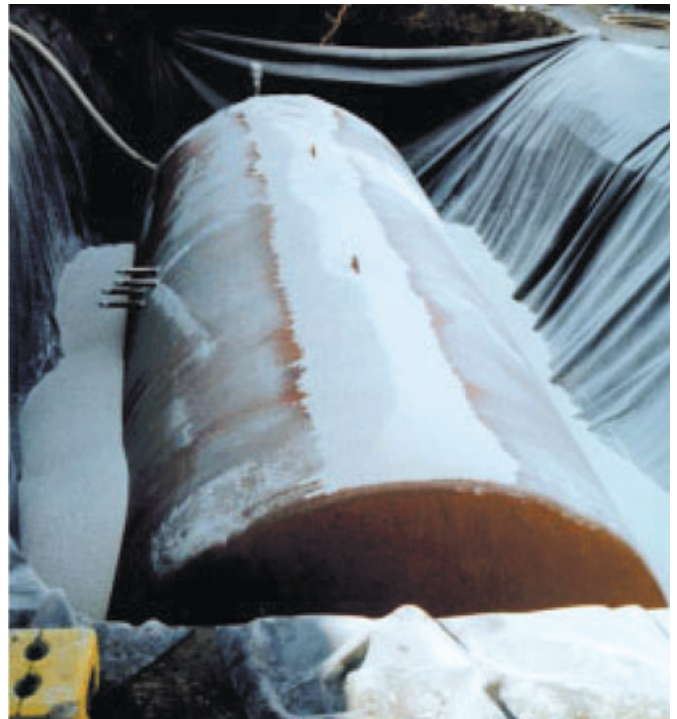
A highly heat-insulating filling with Poraver ensures there is hardly any energy loss in a hot-water tank installed underground in the yard of a trade business in Pfronten.
